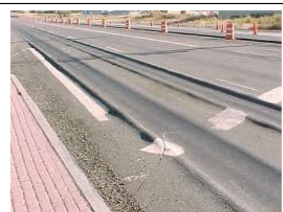
Figure 1. Rutting failure in asphalt pavement
